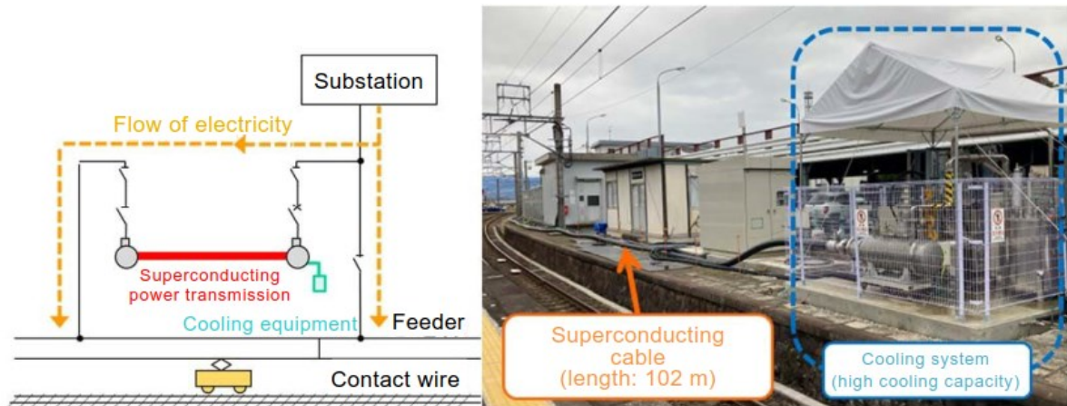
Fig. 1 Overview of Superconducting Feeding System
